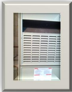
21 HVAC equipment in basement
